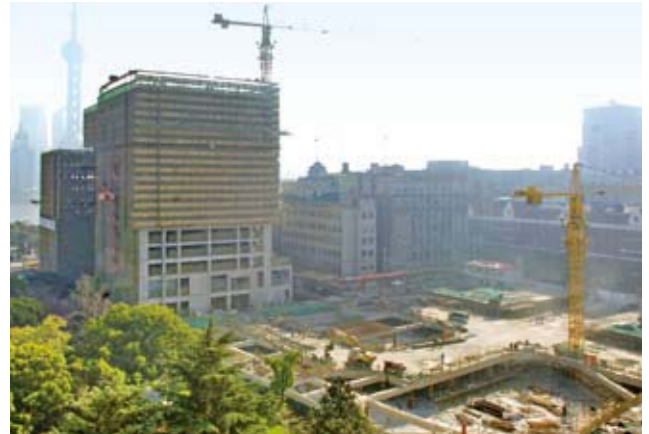
During the year, significant progress was made on the construction of the hotel and hotel apartment tower
